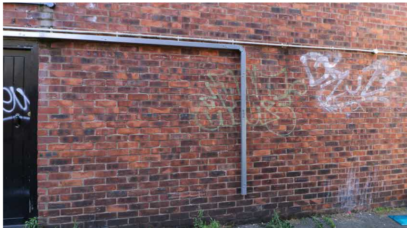
Fig. 3 - Graffiti on the wall
