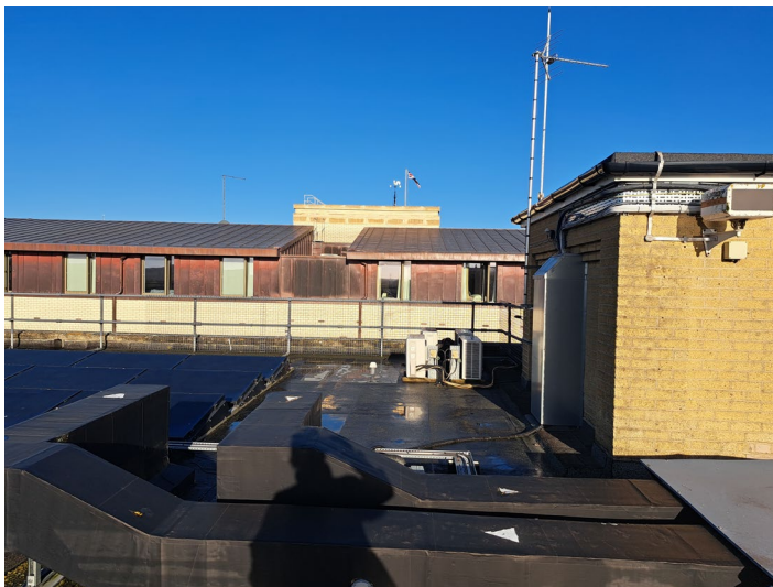
Photos illustrating screening from the north and the set back location of the proposed plant.
