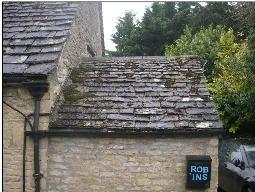
Photograph 3: Rear (Rear (North-East) elevation – existing single-storey Kitchen extension ( to be demolished ) shown
