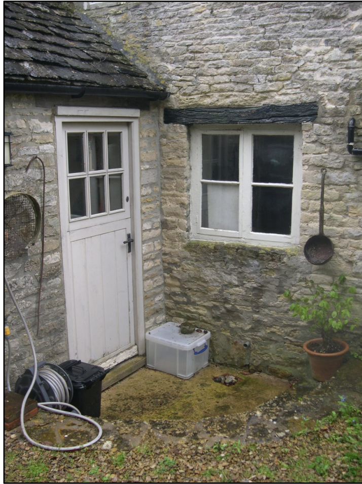
Photograph 4: Front (South-West) elevation of existing Kitchen extension (to be demolished), plus Side (North-West) Ground Floor window
