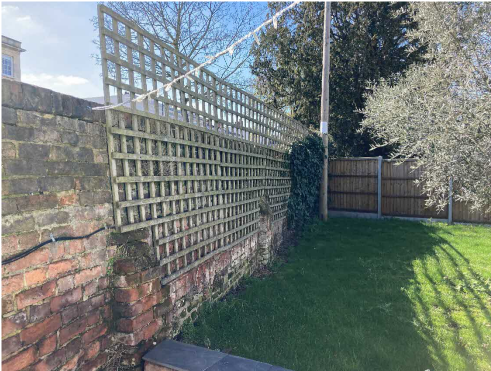
XXVI. Foreground wall leans out towards footpath, background wall leaning in towards garden
