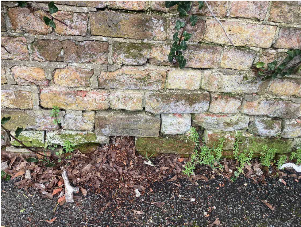
IX. Deterioration of brick at ground level
