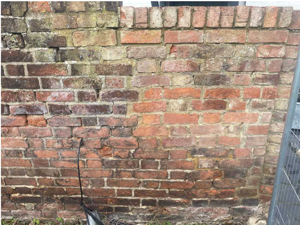
XII. Open cracks running through centre of bricks
