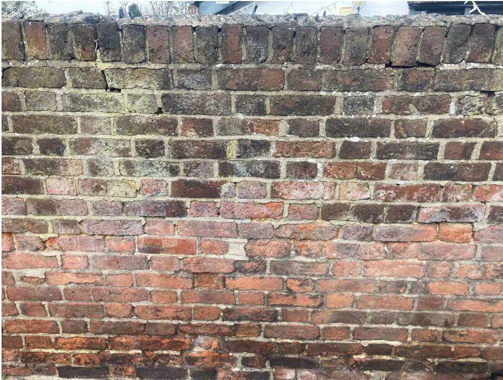
XI. Right of photo above not broken glass and cement capping.
