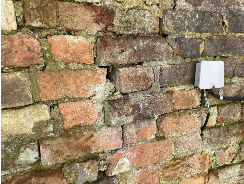
XV. Open crack
