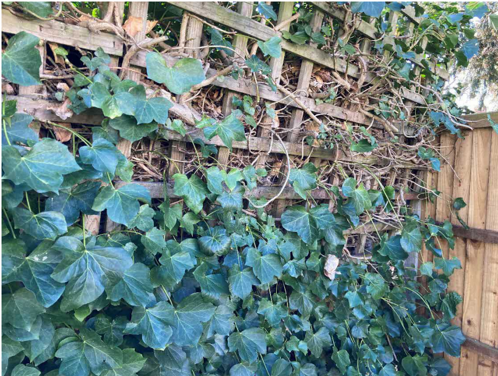
XXI. Trellis and ivy holding wall up
