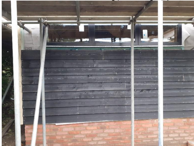
Fig 3. WALLS: Horizontal timber cladding (featheredged), painted black. As installed part-way through construction on the 16 th November 2023
