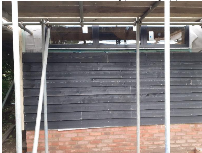
Fig 12. WALLS: Horizontal timber cladding (featheredged), painted black. As installed part-way through construction on the 16 th November 2023
