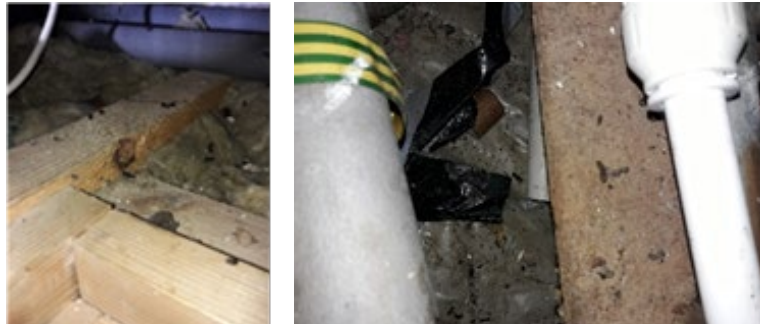
Figure 4. Droppings found within roof voids.
