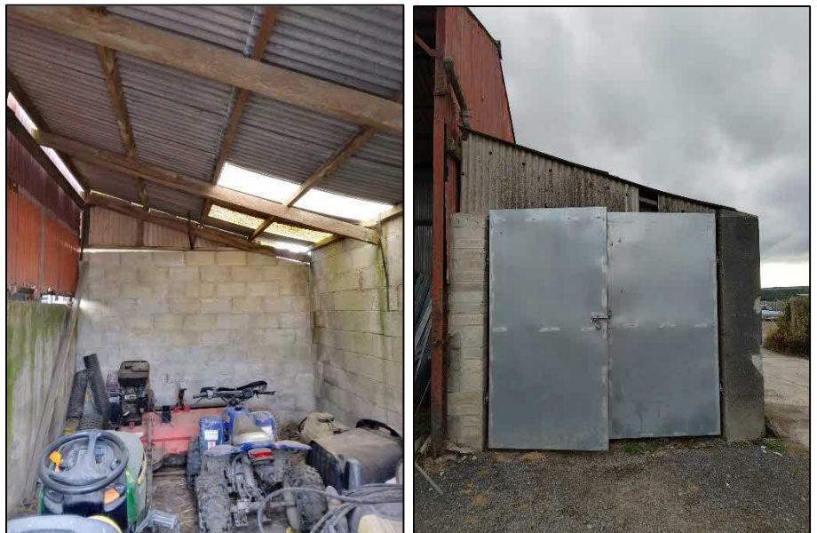
Photos 1 and 2: Internal view of the lean-to extension (left); east face of the extension showing metal double doors (right).
