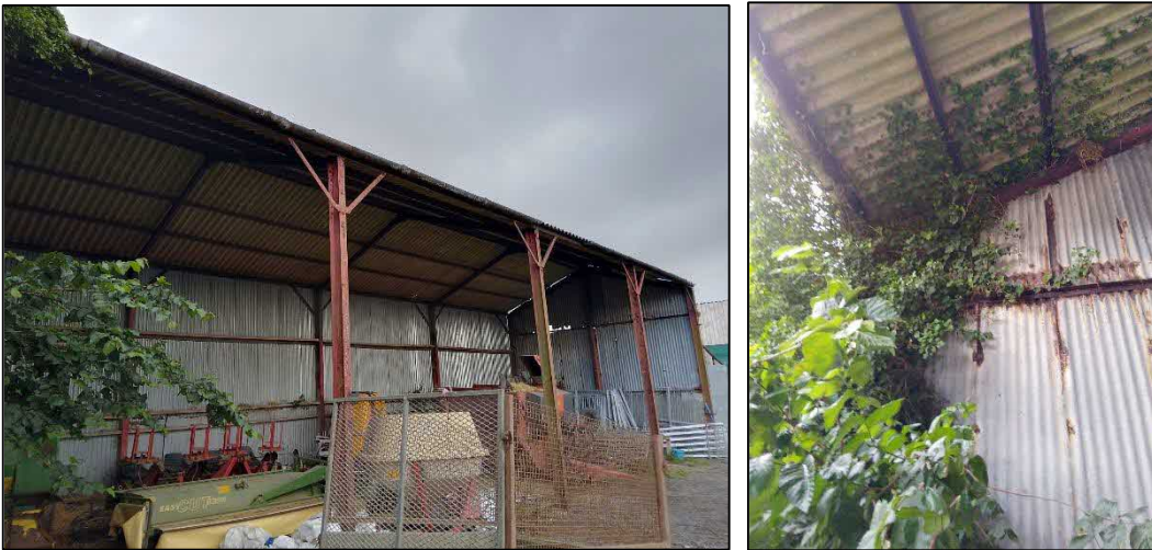
Photos 3 and 4: East face of the main barn; internal south face of the barn.
