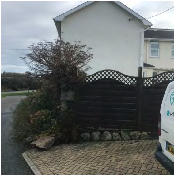
Services - Power overhead into dwelling:
