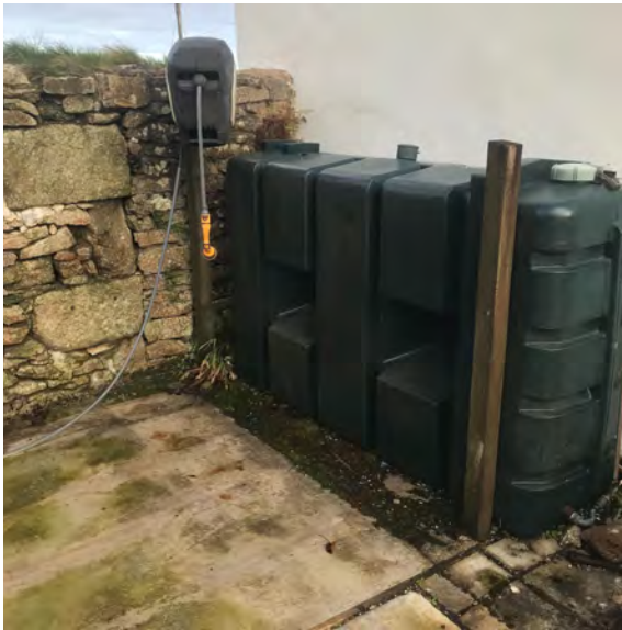
Services - Oil tank:
