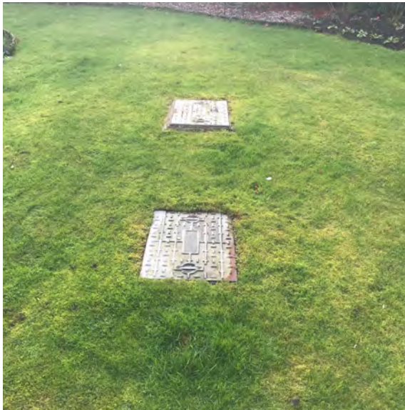
Services - Septic tank in raised lawn:
