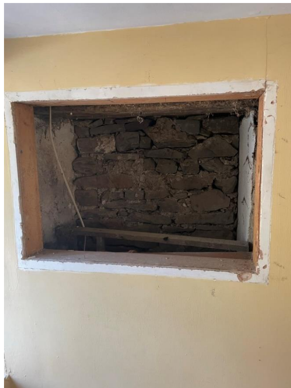
Figures 6-7 – Existing annexe dining room, opening to main sitting room to be reinstated. Photos showing stone in-fill, timber lintels and plastered wall reveals, indicating historic opening, understood to have been blocked up in the 20th Century.
