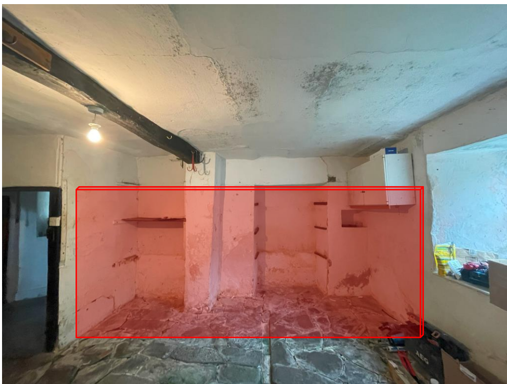
Figure 2 – Existing utility room. New shower and WC to be installed behind bespoke three-quarter timber stall partition on raised floor. Final joinery details to be submitted for approval.
