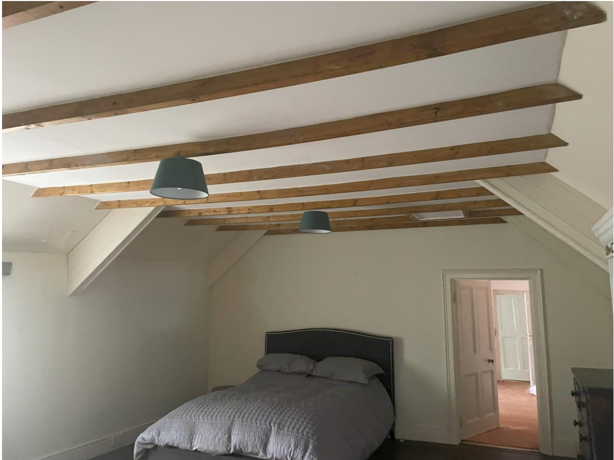
Figure 14 – Bedroom 2 ceiling – plasterboard to be fixed to underside of 20 th Century timber beams, skimmed and painted, to provide ceiling of height and finish consistent with adjacent rooms.
