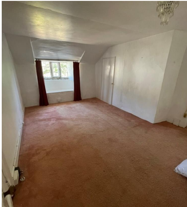
Figure 1 – Existing Bedroom 5 to be converted into a ‘Jack and Jill’ bathroom, retaining the through-passage layout. Pipework to be boxed in at low level and soil pipes to be located within existing cupboard, dropping down into the utility below.
