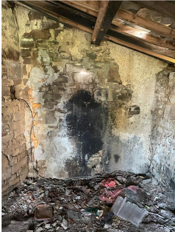
Figure 13 - Interior of lean-to store and location of proposed oil boiler, to be set on concrete plinth. Flue to terminate through rag slate roof. Service pipes to enter main house through blocked up opening (area of blackened render).
