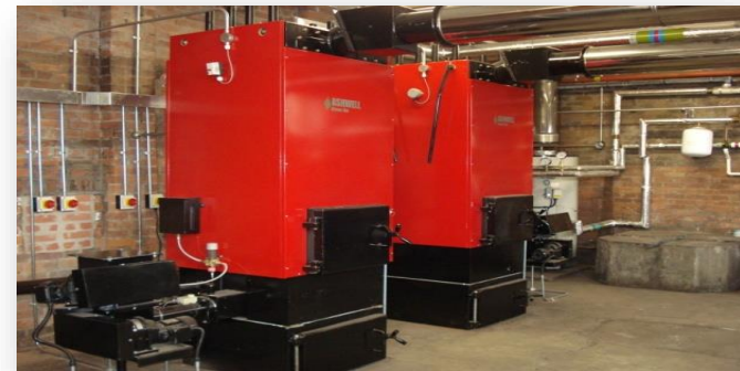
Plantroom Biomass Installation
