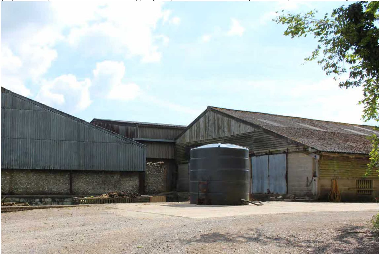
Photograph H. South westerly view. The roofline of the large agricultural buildings to the north of the farmstead can be seen. Part of the fabric of the earlier farm building can be seen to the lower part of the barn to the left, with knapped flint edged with red brick. Modern building materials otherwise comprise of asbestos sheeting to roofs and facades, with part timber cladding of breezeblock wall construction.
