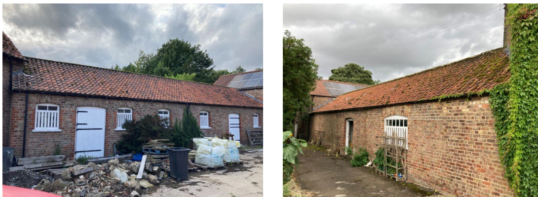
Photograph 2: Representative external views of the Building 2, eastern aspect (left) and western aspect (right).
