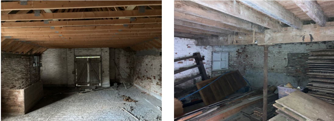
Photograph 4: Representative internal views of Building 3 first floor (left) and ground floor (right).
