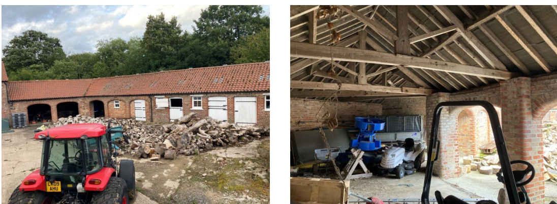
Photograph 5: Representative external view of Building 4 southern aspect (left) and internal view adjacent open waggon bays (right).
