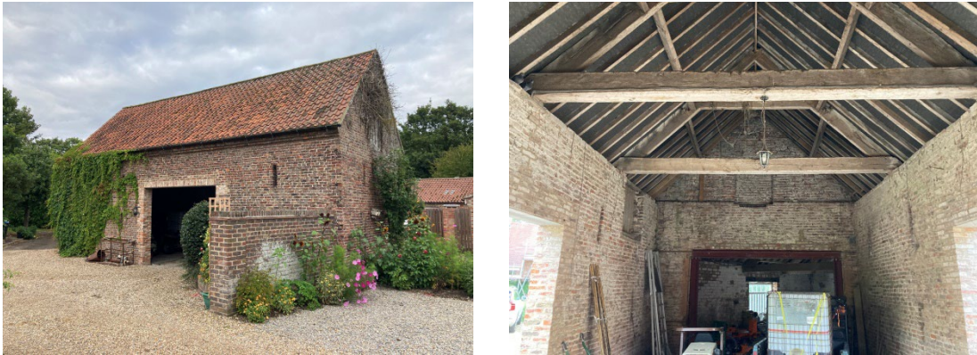
Photograph 1: Representative views of the Building 1, south eastern aspect (left) and internal (right)
