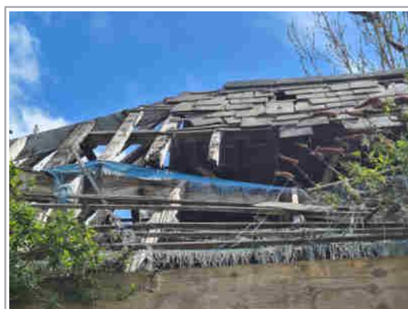
Missing roof covering
