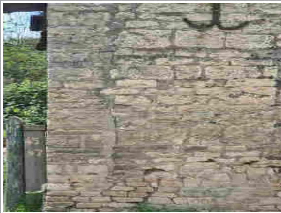
Cracking to north gable
