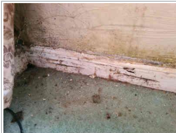
Potential dry rot
