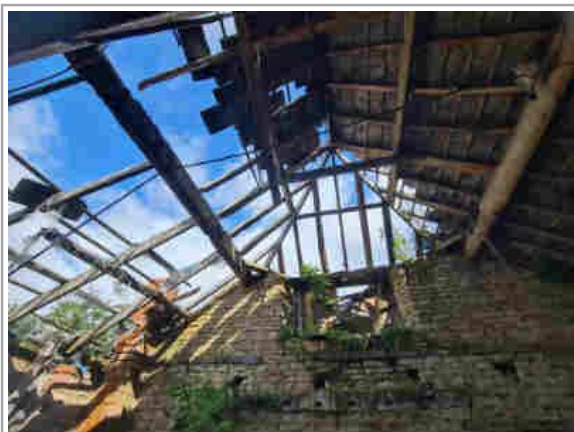
Damaged roof structure
