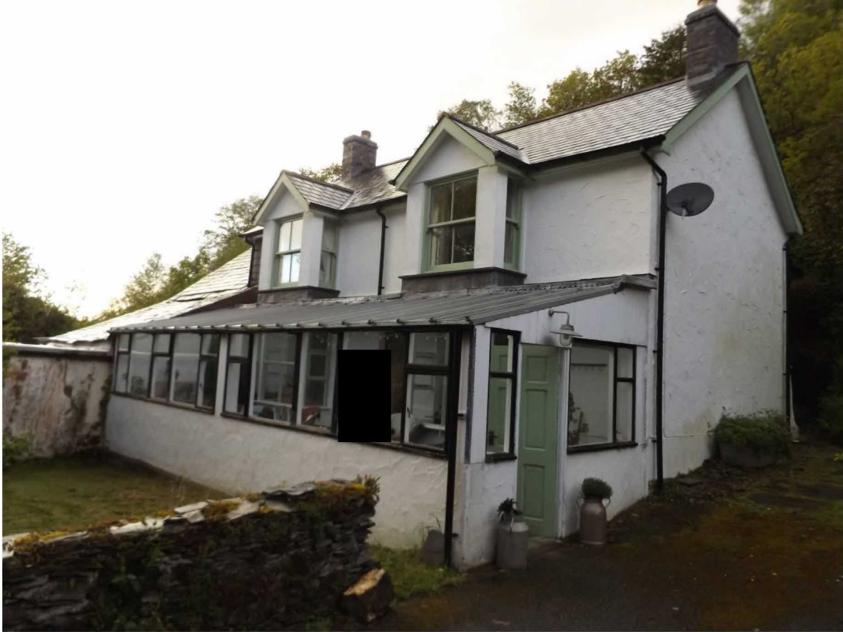
The front elevation of Bwlch y Groes Faen which is in very good condition
