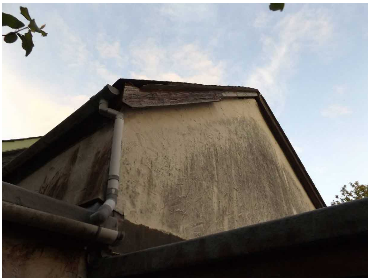
Defects in the edge of the un-renovated roof at the southern end of the building
