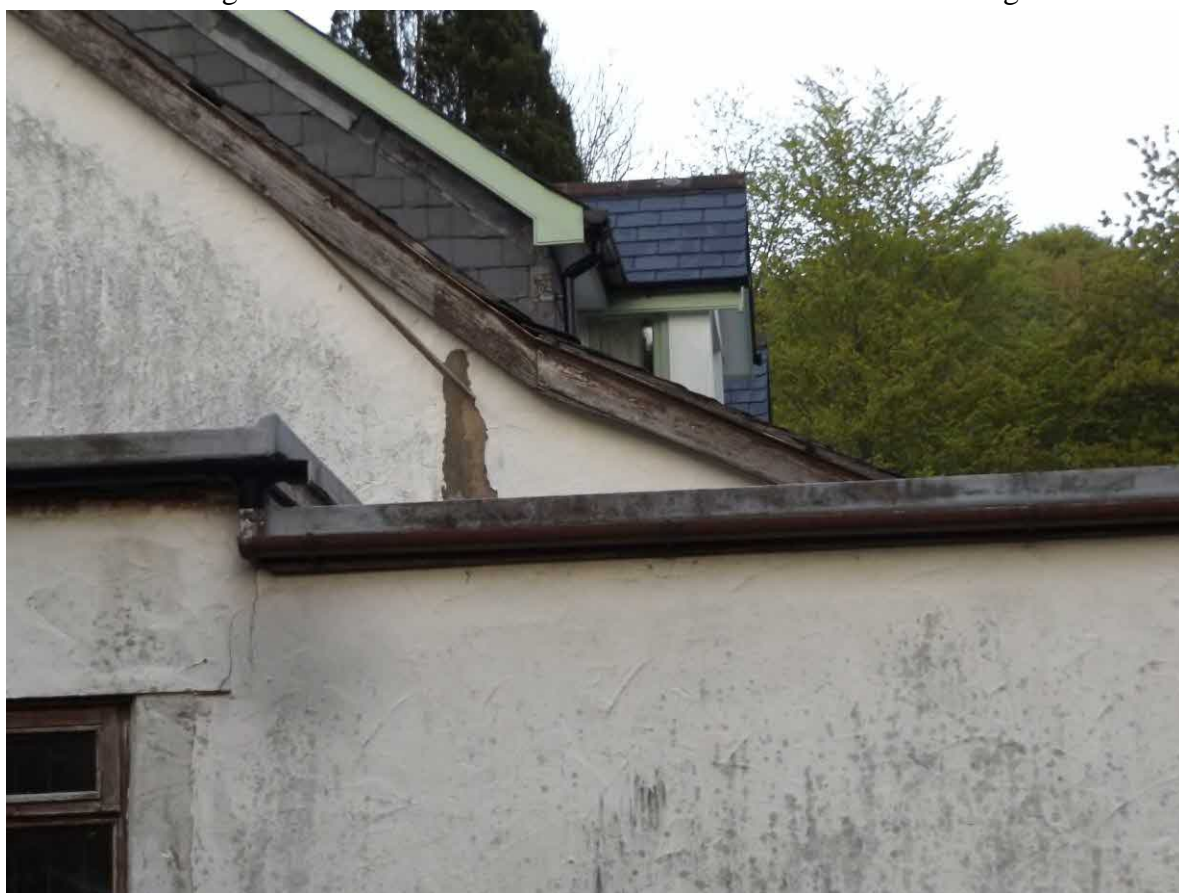
These defects were exploited by pipistrelles
