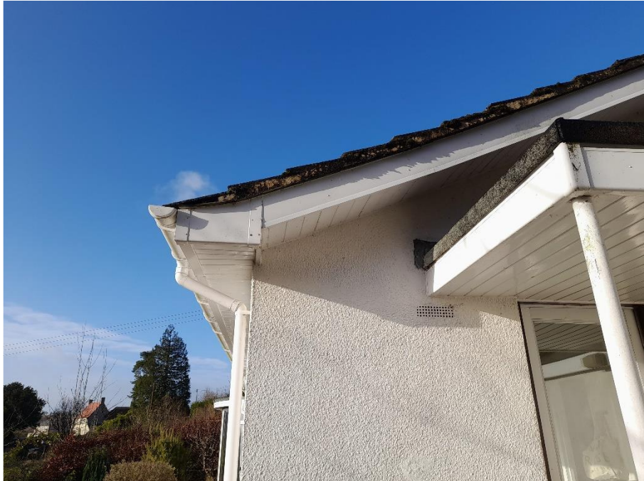
Plate 3 - Crevice under the mortar along the eastern elevation of the house
