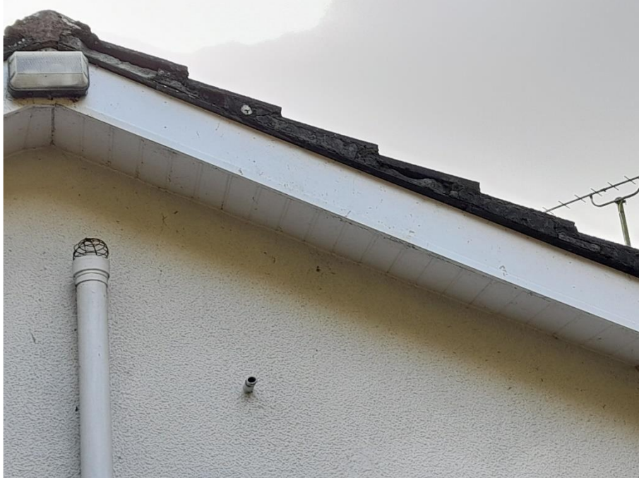
Plate 2 - Crevices under the mortar along the western elevation of the house
