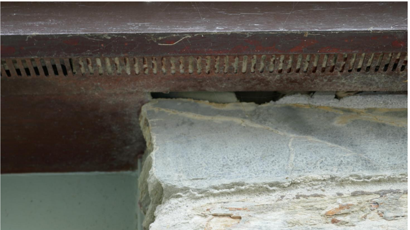
Figure 8. Gap present at the wall top of the garage.
