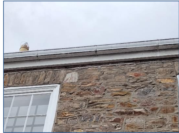
Holes at wall tops to front of building
