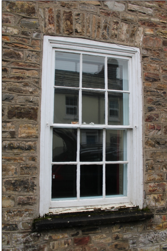
Plate 12: View of ground-floor window in the main façade showing the form of the window, internal secondary glazing and areas of damage
