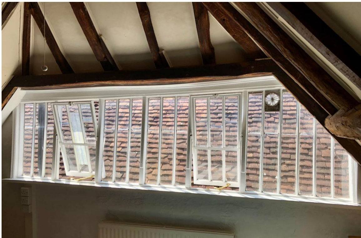
Fig 4: The west facing side window dates from the early 20 th Century and contains an ad-hoc design made up of timber and metal. The proposal would replace this with a quality design using timber joinery and slimline glazing.
