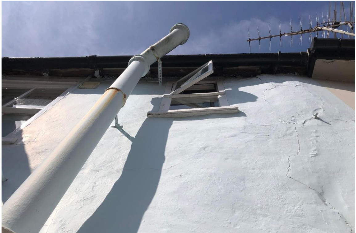
Fig 3: On the rear elevation of the building, the small stair window is believed to have been added at a later date and its fabric dates from the 20 th Century. The proposal would emulate the sash seen to the far left.
