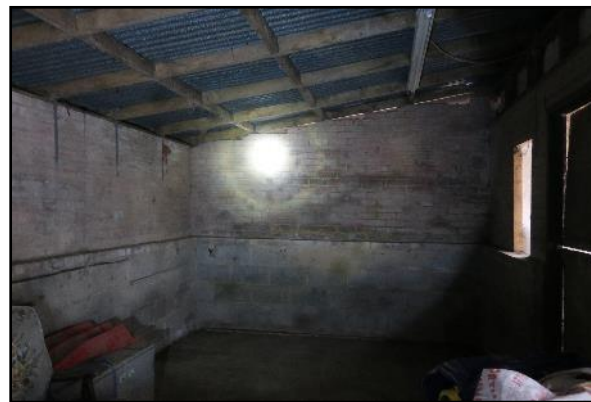
Plate 4: Showing a typical internal view of the Stable Block to the south.
