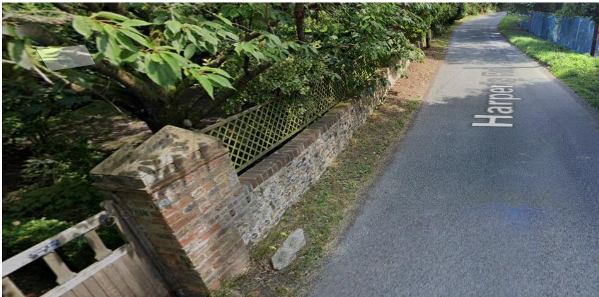
View looking southwards down Harpers Road, a little further down Harpers Road, showing the brick wall, pedestrian gate and then stone wall with iron railings above – Image date 2019 Courtesy and copyright ©Google 2021
