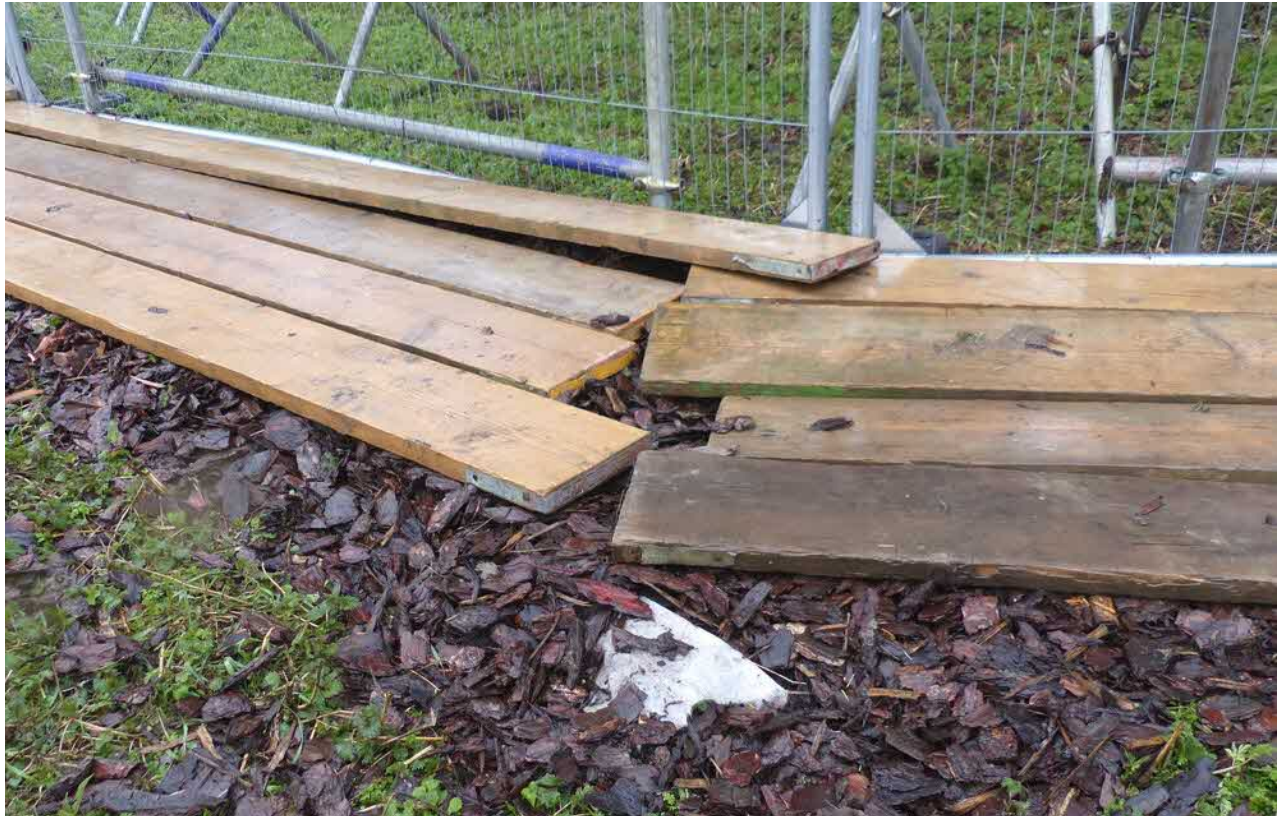
Fig 3. Scaffold boards on top of wood chips serving as ground protection. Note the geotextile layer underneath
