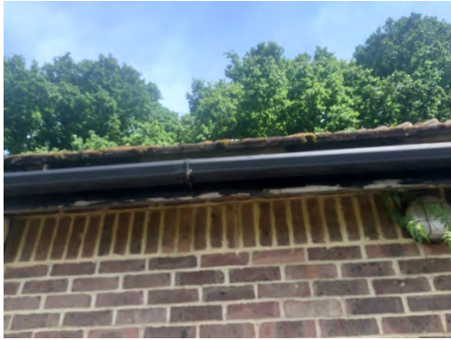
Photo 7. Pool House, Gaps under soffit
