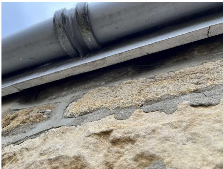
Plate 8. Crevice between fascia board and stonework.
