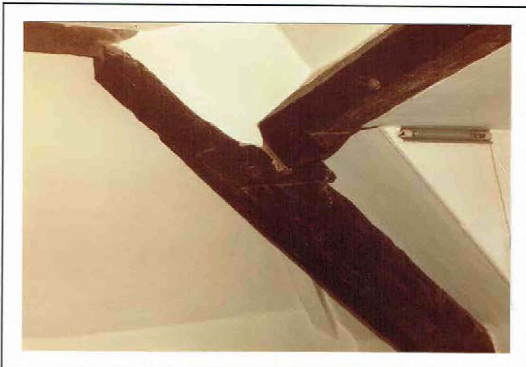
Corner diagonal beam in second bedroom, free of the roof structure: put there possibly because the window gable beam was not long enough to reach the opposite wall. Even then the joint seems to have been botched with an inserted cradle.
