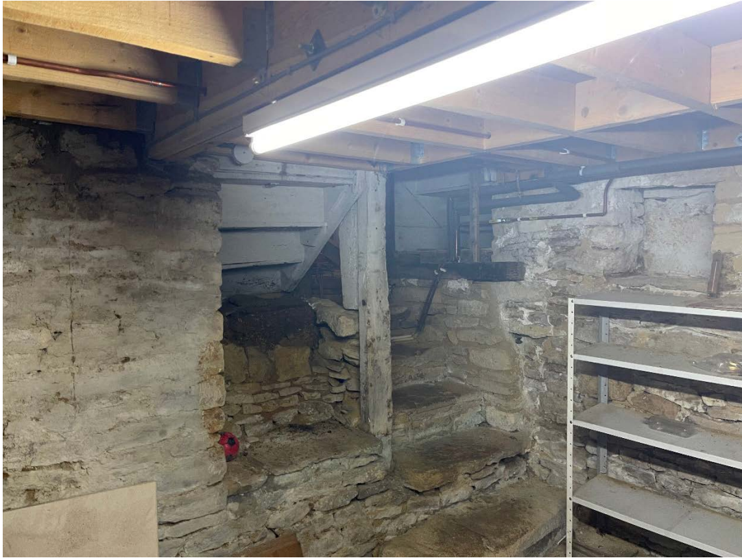
View of existing staircases in basement (note construction joint from C18 extension)
