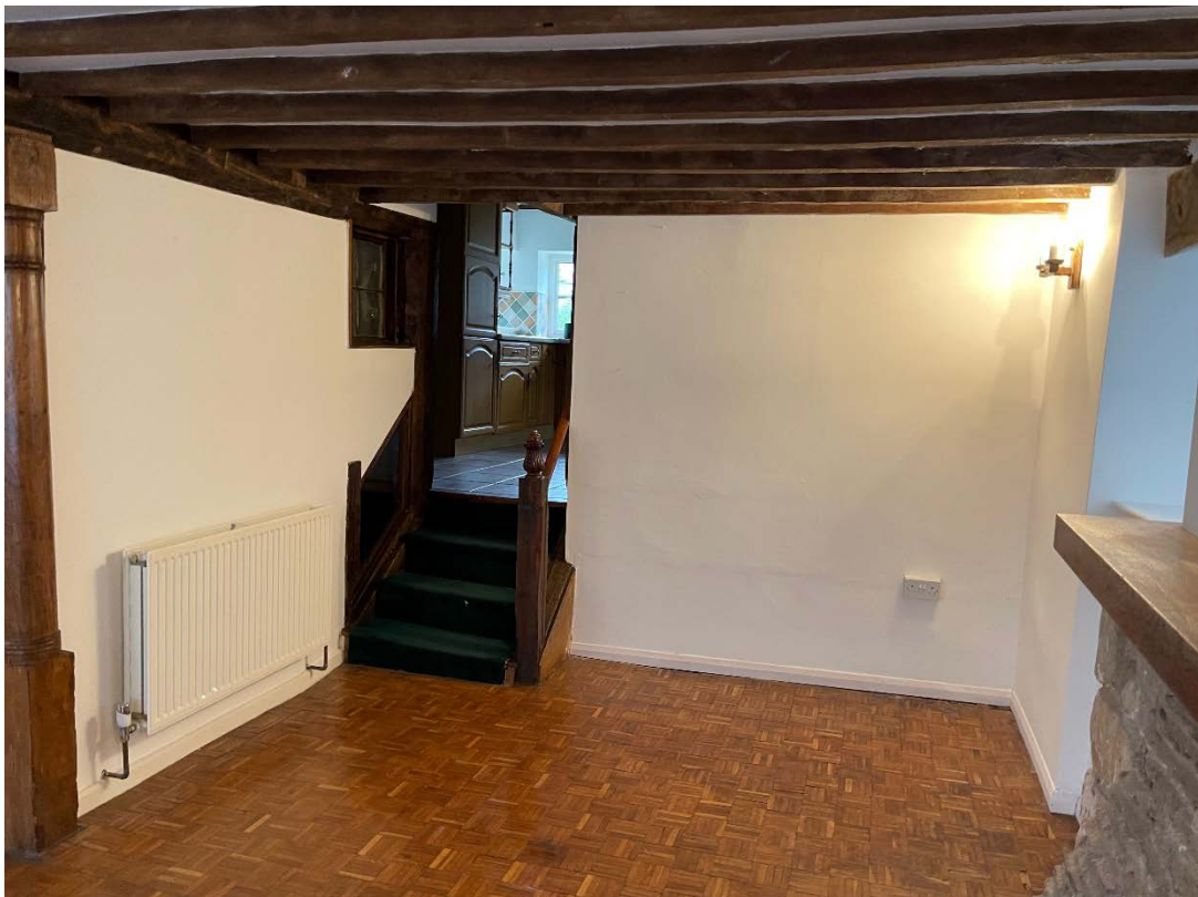
View of existing internal entrance to kitchen (the hollow partition is to be removed)
