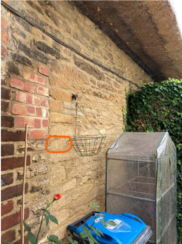
View of construction joint between C17 house & C18 extension from neighbouring garden (note 's' scribed in stone – please refer to 'A story of a house')
