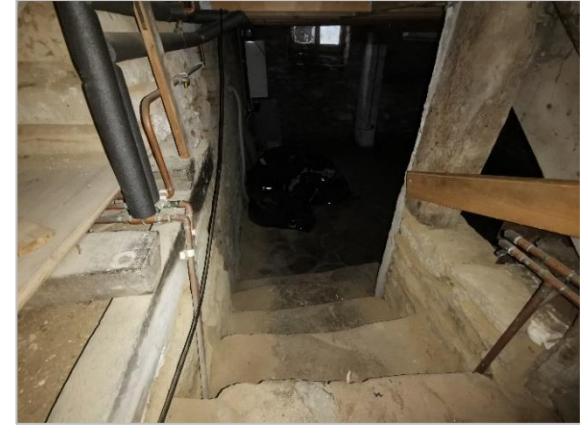
9. Basement stairwell. The vertical timber support to the partition wall above is anachronistic and purportedly supports only the broom cupboard above.
