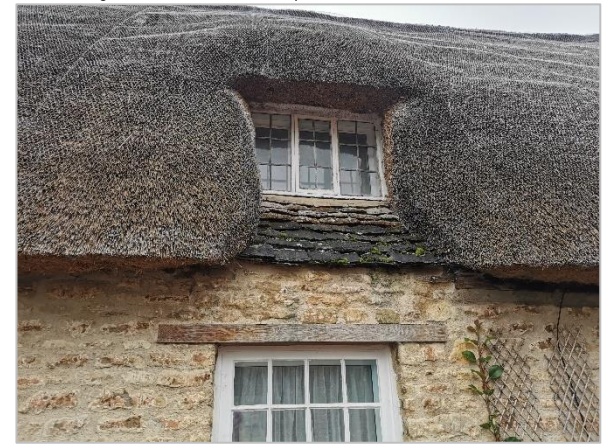
12. Example of Stonesfield slates built into historic sill at front of the Site.
