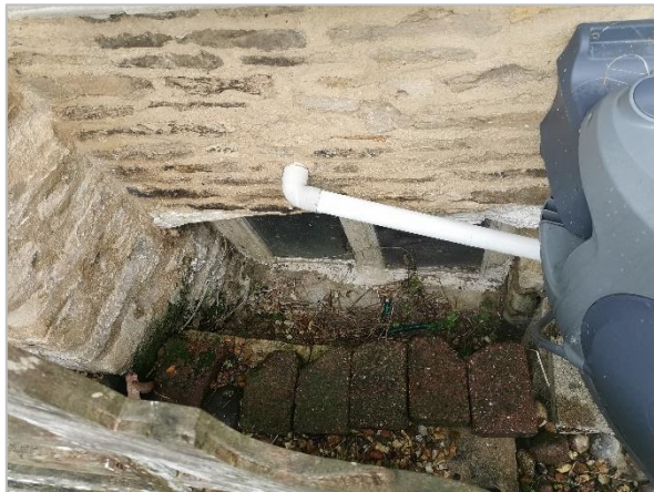
10. Viewing window to cellar. It is unlikely that the cellar was designed to be accessed from the rear of the property, indicating the internal stairwell is contemporary to the cellar as the main access.
