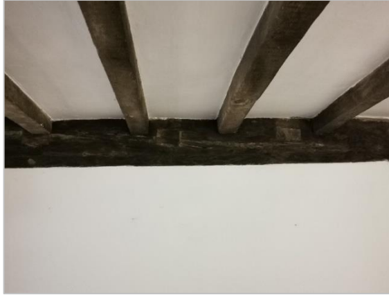
8. Evidence of removal of historic joists and replacement and re-notching of new timber
