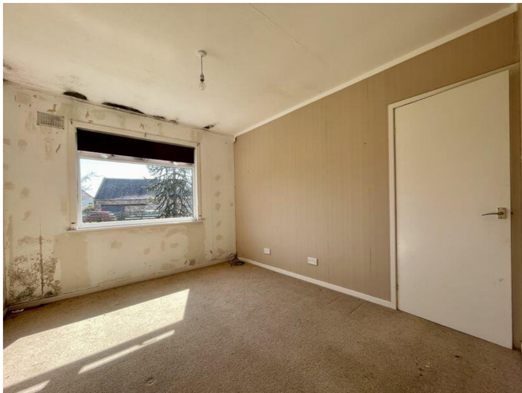
Fig.05 Interior view of Master bedroom with damp/water ingress to walls and ceiling
