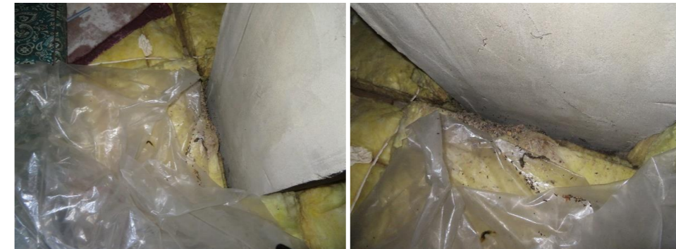
Bat droppings adjacent to disused chimney
