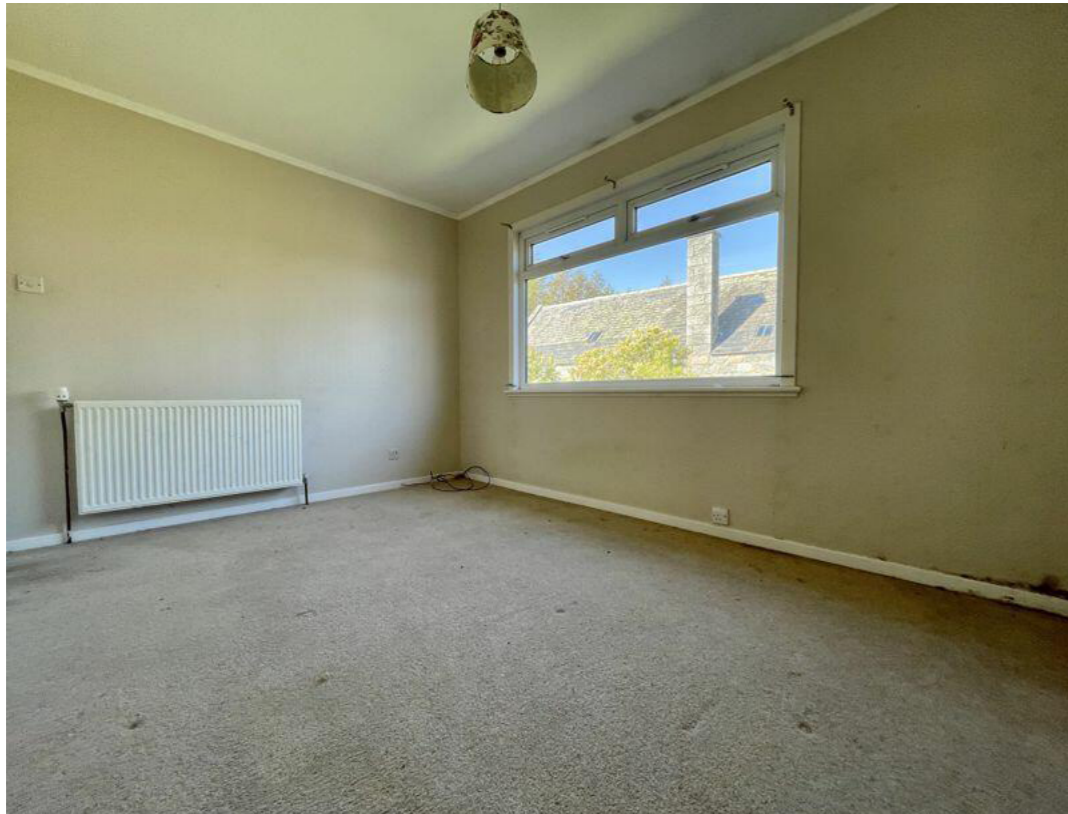
Fig.04 Interior view of sitting room with evidence of damp ingress and mould to the wall and junction with ceiling
