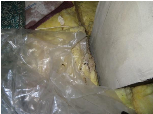
Bat droppings adjacent to disused chimney
