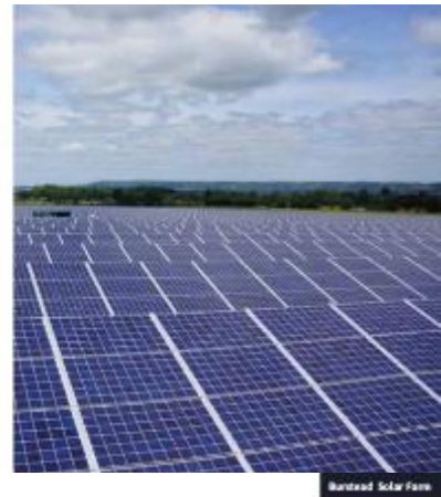
Burstead Solar Farm
