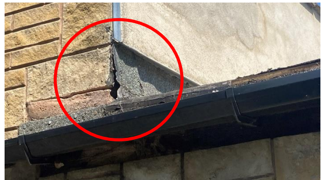
Photo 12: Gap in the roofing felt present building 2.
