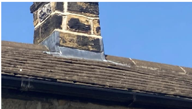
Photo 9: Gaps in the tiles on building 1.
