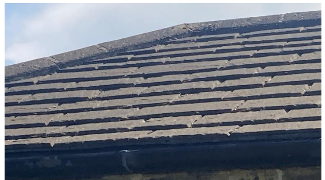
Photo 10: Innumerable gaps on buildings 1 and 3.
