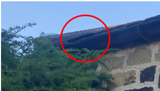
Photo 11: Large gap in tile on building 1
