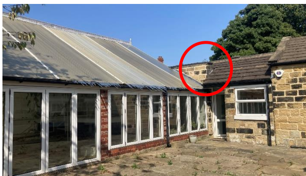
Photo 13: The summer house connected to the cottage, with the large gap present where the buildings meet.
