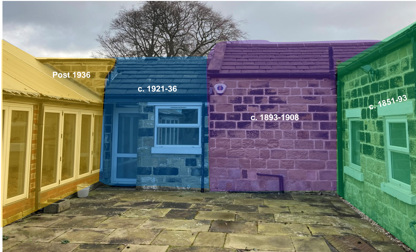
Img 16 – View between The Cottage and Summerhouse patio looking east, providing an overview of parts of the building built in phases at different periods with poorly matched materials.
