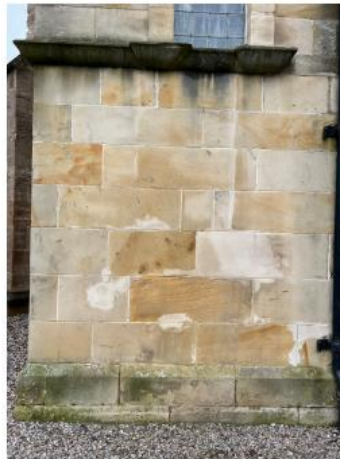
29. Bosh/failed isolated repairs to areas require old repairs to be removed and re done using MM Repair.
