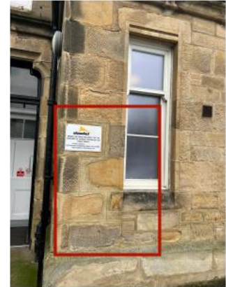
3. Bosh/failed repairs to Dressed ashlar require old repairs to be removed and re done using MM Repair.
