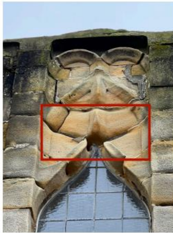
32. Eroded feature stones required replacements & repairs to surrounding stones using MM Repair.
