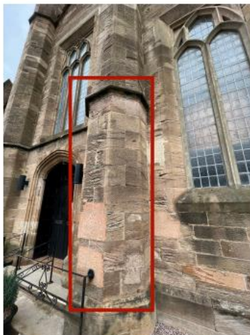
23. Bosh/failed repairs to Dressed buttress require old repairs to be removed and re done using MM Repair.
