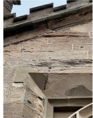
27. Damaged/cracked lintel requires resin anchor stitch repair & full lintel repair.
