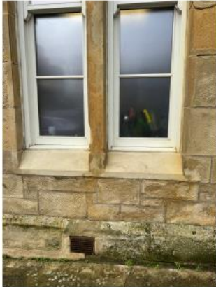
1. Bosh/failed repairs to cills required old repairs to be removed and re done using MM Repair.
