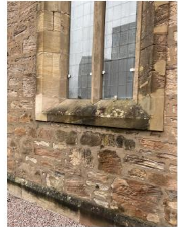
9. Bosh/failed repairs to cills require old repairs to be removed and re done using MM Repair.
