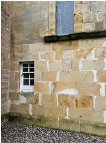
31. Bosh/failed isolated repairs to areas require old repairs to be removed and re done using MM Repair.
