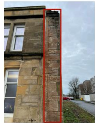
6. Cementitious old repairs to be removal and re done using MM Repair followed by isolated lime pointing to open areas.
