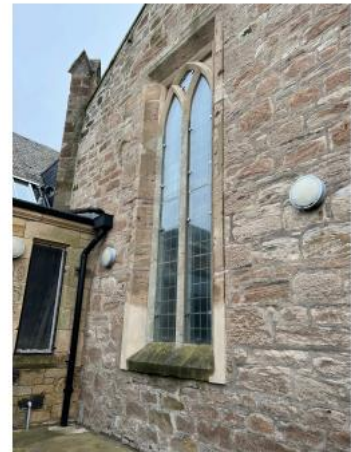
36. Bosh/failed repairs to areas around window require old repairs to be removed and re done using MM Repair.
