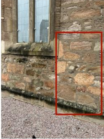
13. Bosh/failed isolated repairs to areas around base of section F require old repairs to be removed and re done using MM Repair.
