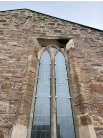
35. Bosh/failed repairs to areas around window require old repairs to be removed and re done using MM Repair.
