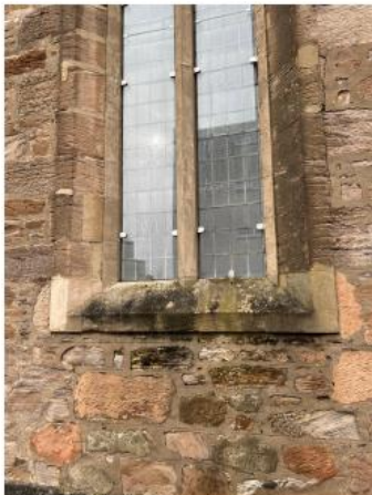
10. Bosh/failed repairs to cills require old repairs to be removed and re done using MM Repair.
