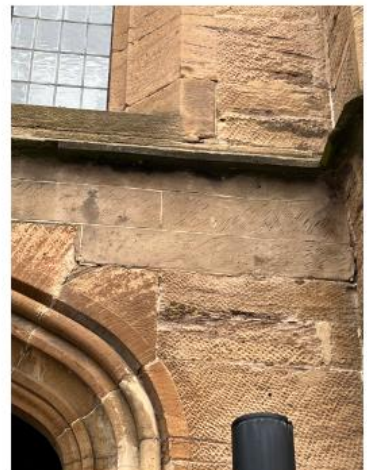
24. Bosh/failed repairs to Dressed ashlar require old repairs to be removed and re done using MM Repair.
