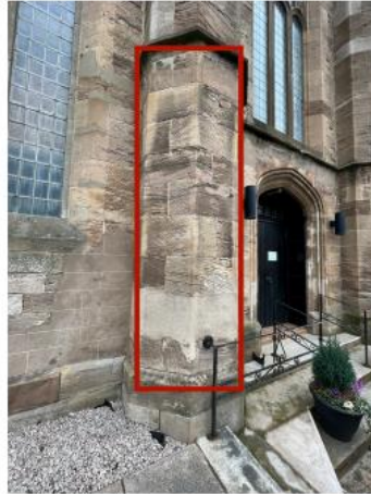
26. Bosh/failed repairs to Dressed buttress require old repairs to be removed and re done using MM Repair.
