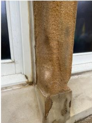
4. Base of Mullion has weathered and requires part repair using MM Repair.
