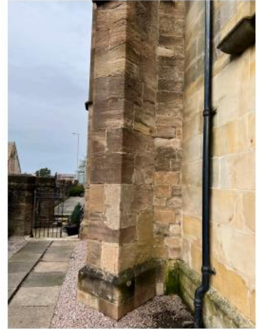
21. Cementitious old repairs to be removal and re done using MM Repair.
