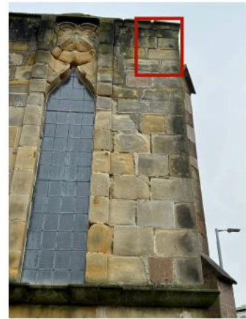
33. Top corner requires 3 courses to be striped following movement and rebuild using sufficient ties.
