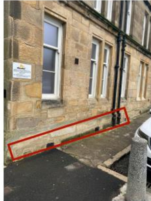
2. Bosh/failed repairs to plinth course require old repairs to be removed and re done using MM Repair.
