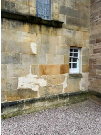
19. Bosh/failed isolated repairs to areas around base of section E require old repairs to be removed and re done using MM Repair & resin anchor stitch repair
