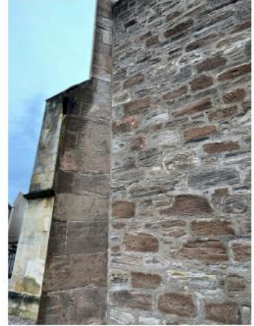
15. Isolated thin bosh repairs require redressed/removed and carborundum rub.
