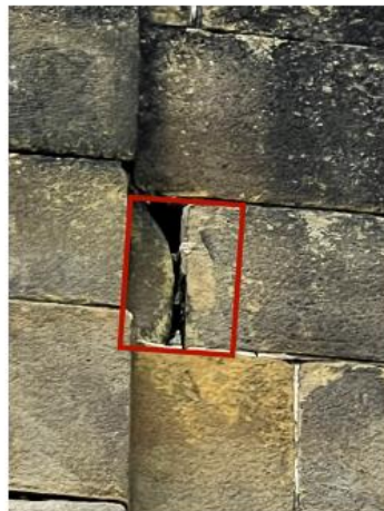
17. Stone replacement required to damaged dressed ashlar section.
