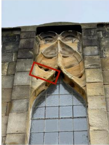
20. Eroded feature stone required replacement & repairs to surrounding stones using MM Repair.
