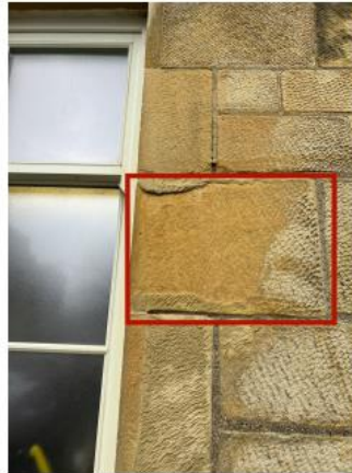
5. Bosh repairs have failed around window rybat, stone requires a redress and partial repair.
