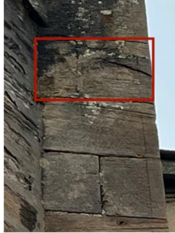
14. Stone replacement required to damaged quoin section.
