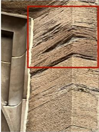
25. Isolated part repair required to window rybat to avoid water build up.
