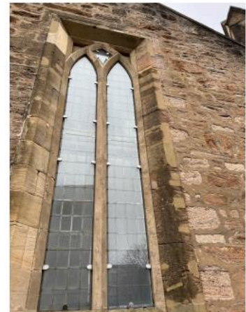
12. Bosh/failed repairs to areas around window require old repairs to be removed and re done using MM Repair.
