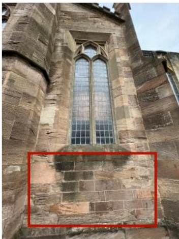
22. Bosh/failed repairs to Dressed ashlar require old repairs to be removed and re done using MM Repair.
