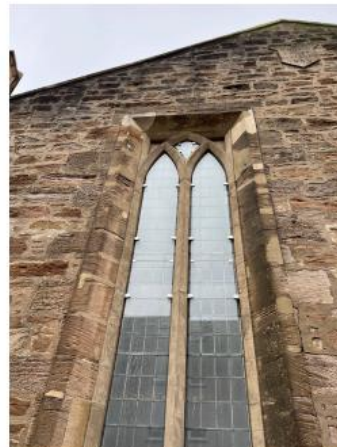
11. Bosh/failed repairs to areas around window require old repairs to be removed and re done using MM Repair.
