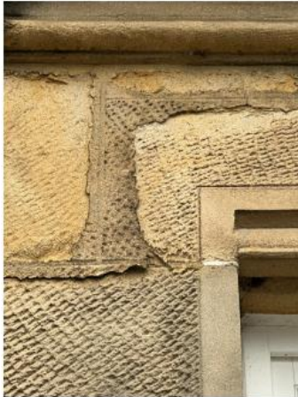
7. Bosh/failed repairs to lintels require old repairs to be removed and re done using MM Repair to 4 areas market in Section G.
