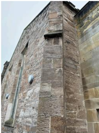
34. Bosh/failed repairs to Dressed buttress require old repairs to be removed and re done using MM Repair.
