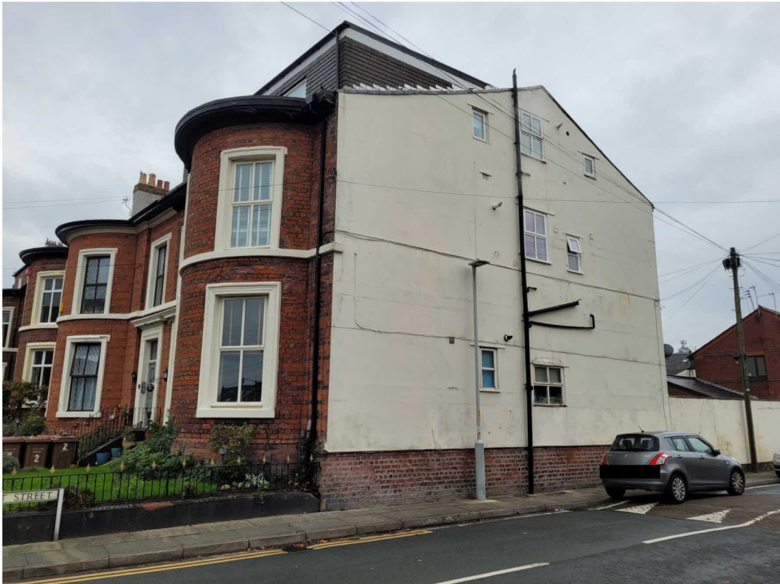
SIDE ELEVATION – TWO GROUND FLOOR WINDOWS TO BE REPLACED AND LINTELS REPAIRED AS NECESSARY
