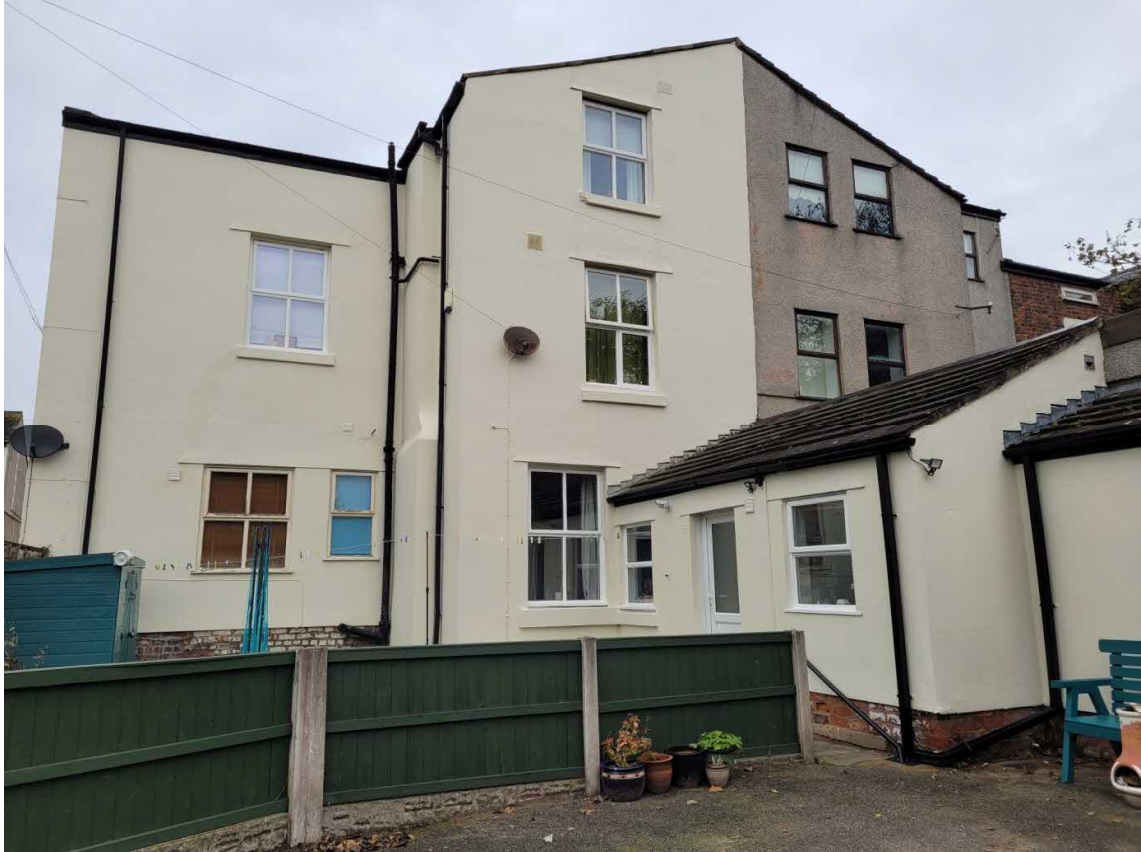
REAR ELEVATION – TWO GROUND FLOOR WINDOWS TO BE REPLACED AND LINTELS REPAIRED AS NECESSARY
