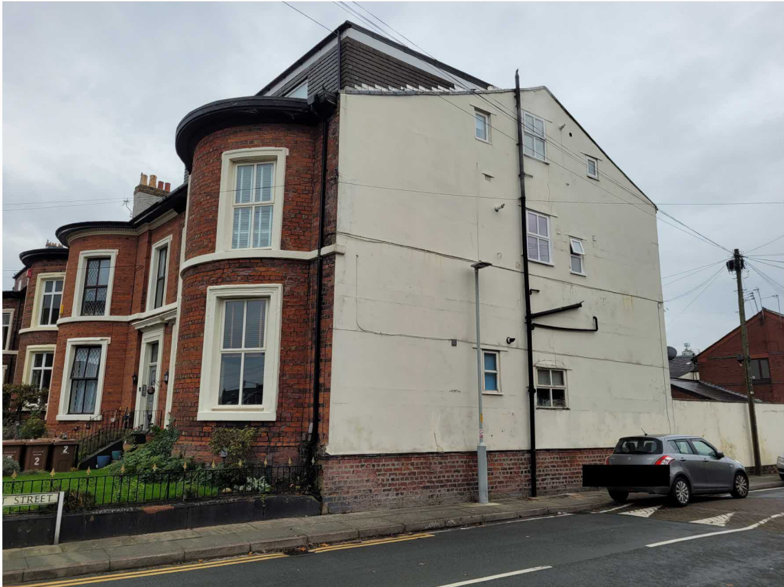
SIDE ELEVATION – TWO GROUND FLOOR WINDOWS TO BE REPLACED AND LINTELS REPAIRED AS NECESSARY
