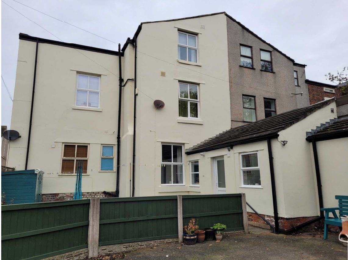
REAR ELEVATION – TWO GROUND FLOOR WINDOWS TO BE REPLACED AND LINTELS REPAIRED AS NECESSARY
