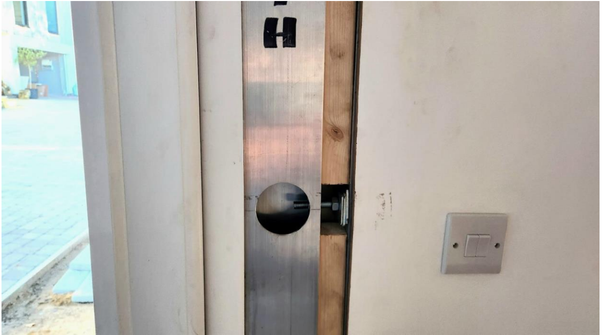
Bolts connecting two halves with access panel for tightening
