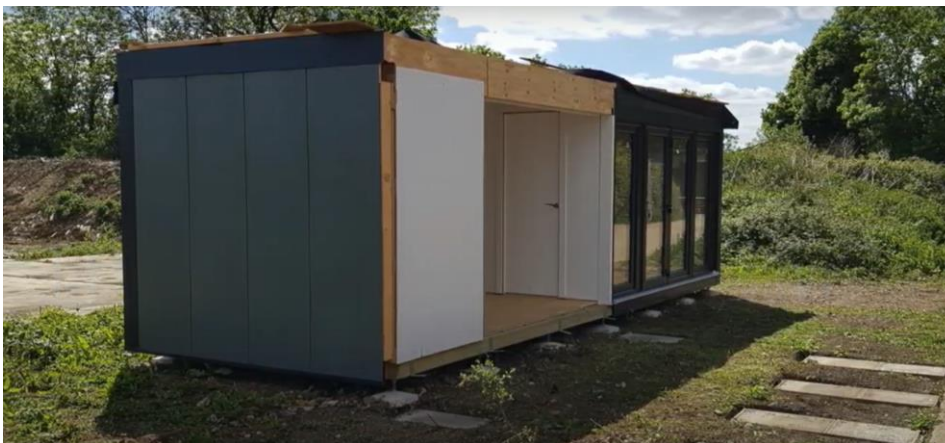
First part in place, note shallow padstones in place in readiness for second part.
