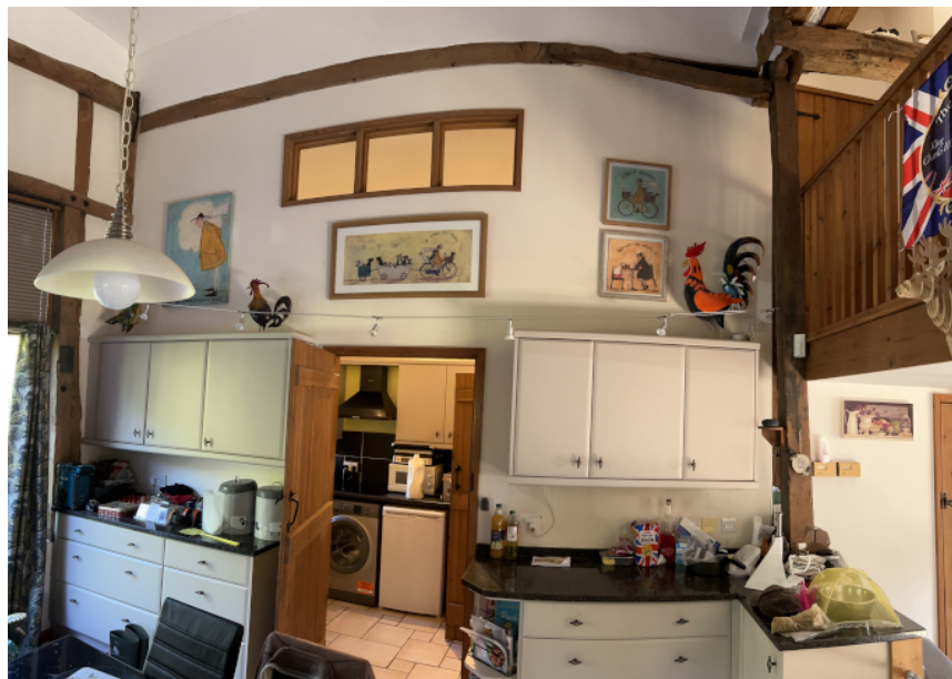
Plate 6 - Wall between R002 & R007/R008. R007 & R008 are formed within an extension to the original barn with historic framing visible in all other partitions except that which is proposed to be removed.
