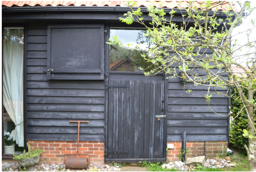
Plate 3 - Glazed panel to be replaced. Outer frame including upper and lower stable doors retained.
