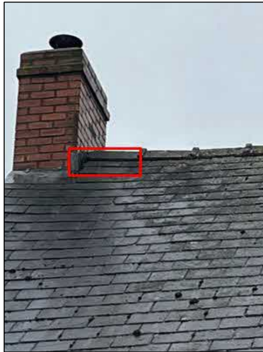
Plate 12. Gaps under ridge tile and around chimney
