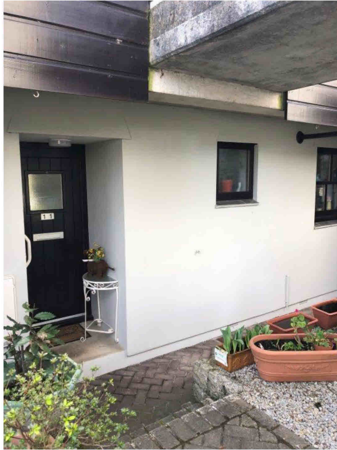
Figure 6 – Photograph showing existing single glazed door on the central flat complex.
