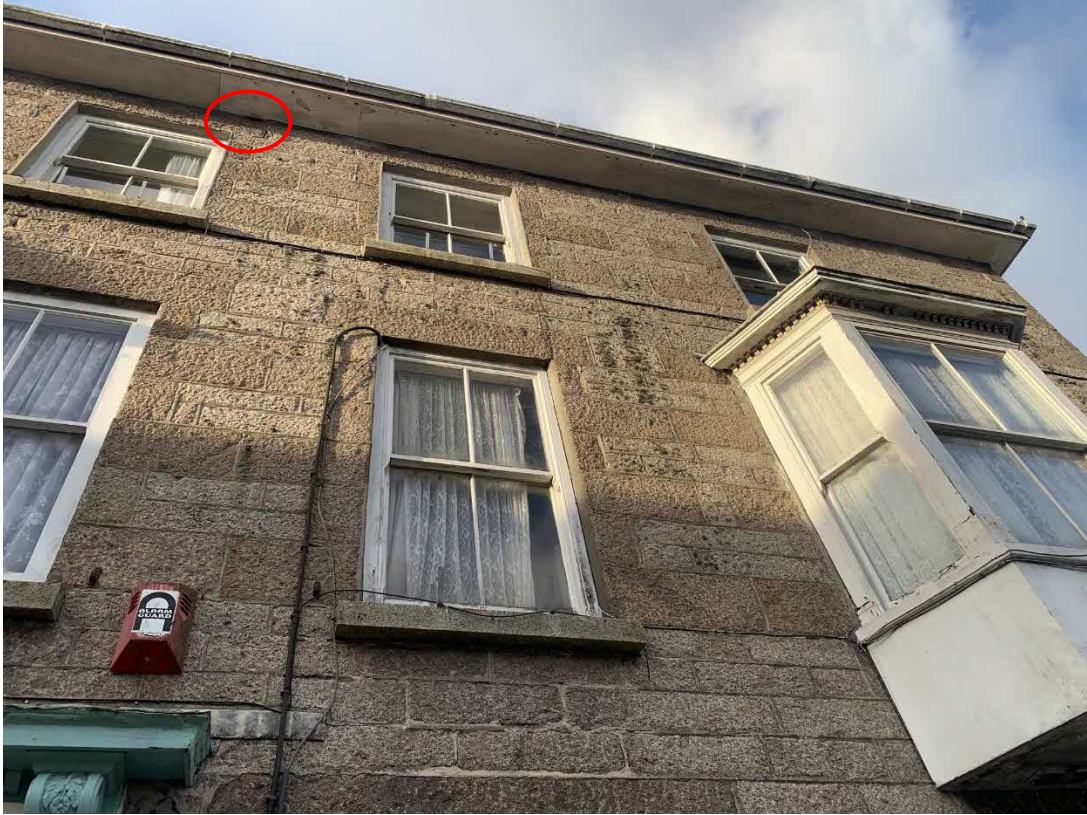
Figure 2: Gap in soffit
