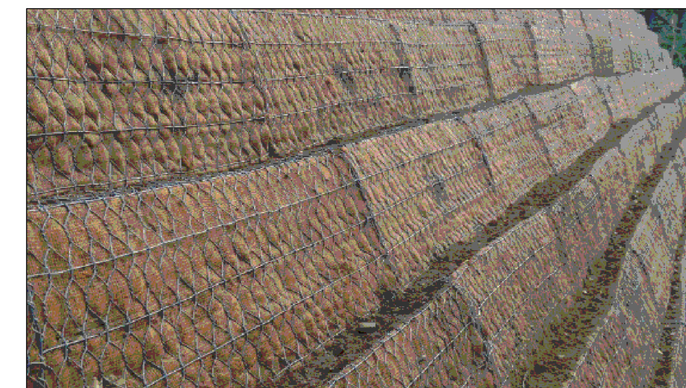
TYPICAL PHOTO OF "MACCAFERRI GREEN TERRA MESH" RETAINING STRUCTURE PRIOR TO VEGETATION ESTABLISHING
