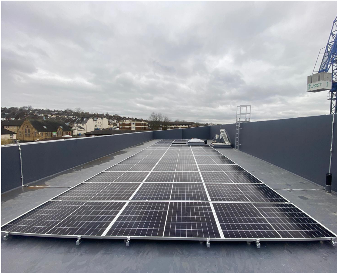
Picture of mechanical fixed Nicholson IFP Solar PV Installation undertaken by Envirolec – Yeoman House, Rochester
