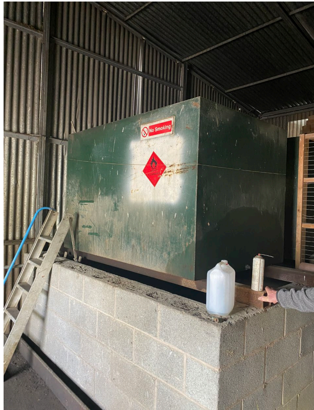
Photograph 25: Bulk fuel storage tanks in use in main workshops on Site
