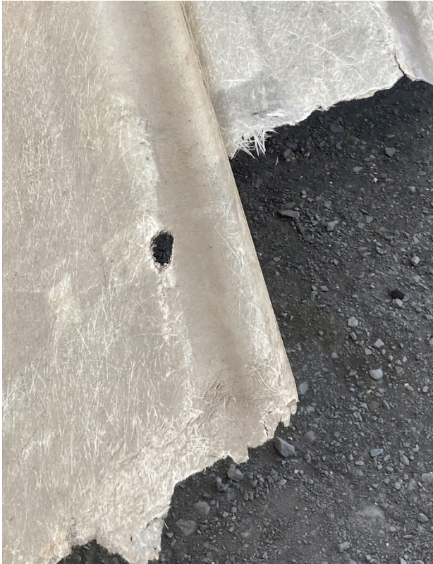
Photograph 19: Potentially asbestos containing material located adjacent to the main workshops in the centre of the Site
