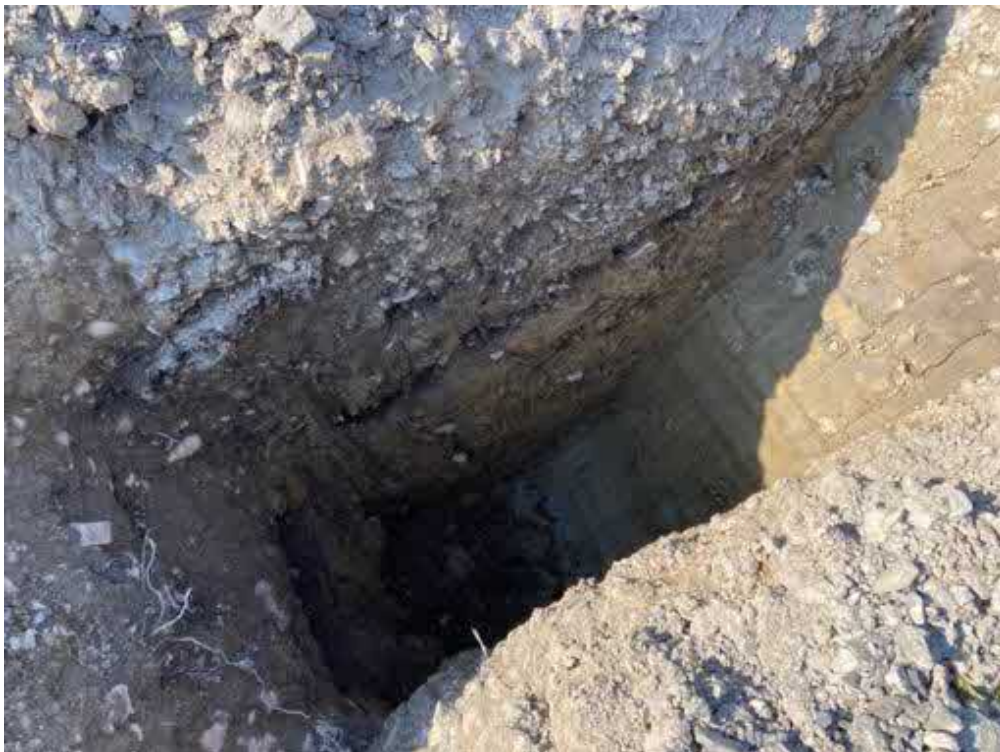
Photograph 54 Description: Trial pit TP24 Date: 07/06/2023 Location: Lay down area in the north-western part of the Site
