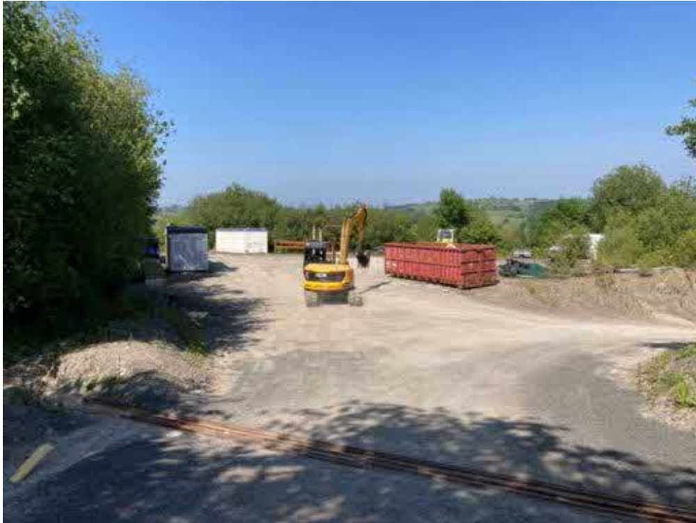
Photograph 53 Description: Lay down area (between lower and middle quarry benches) Date: 07/06/2023 Location: North-western part of the Site – looking to the north
