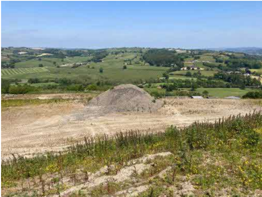
Photograph 33 Description: Central part of middle bench (incl. stockpile of imported material) Date: 07/06/2023 Location: Central-southern part of the Site – looking to the north-east
