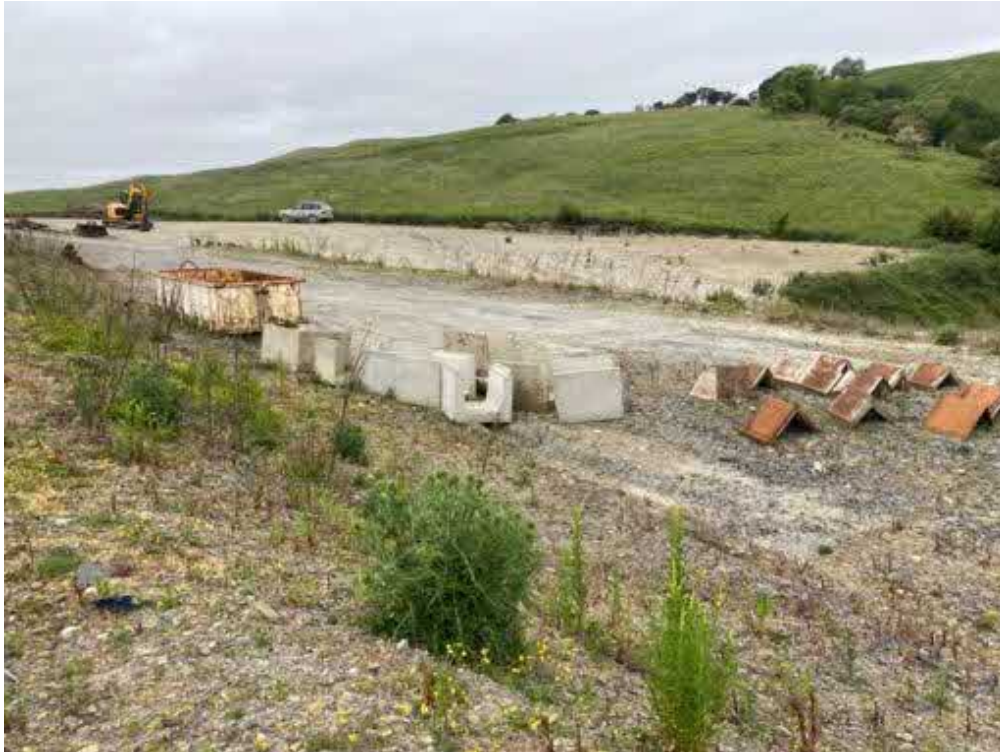
Photograph 11 Description: Storage of miscellaneous materials on upper bench Date: 07/06/2023 Location: South-western part of the Site – looking to the north-west
