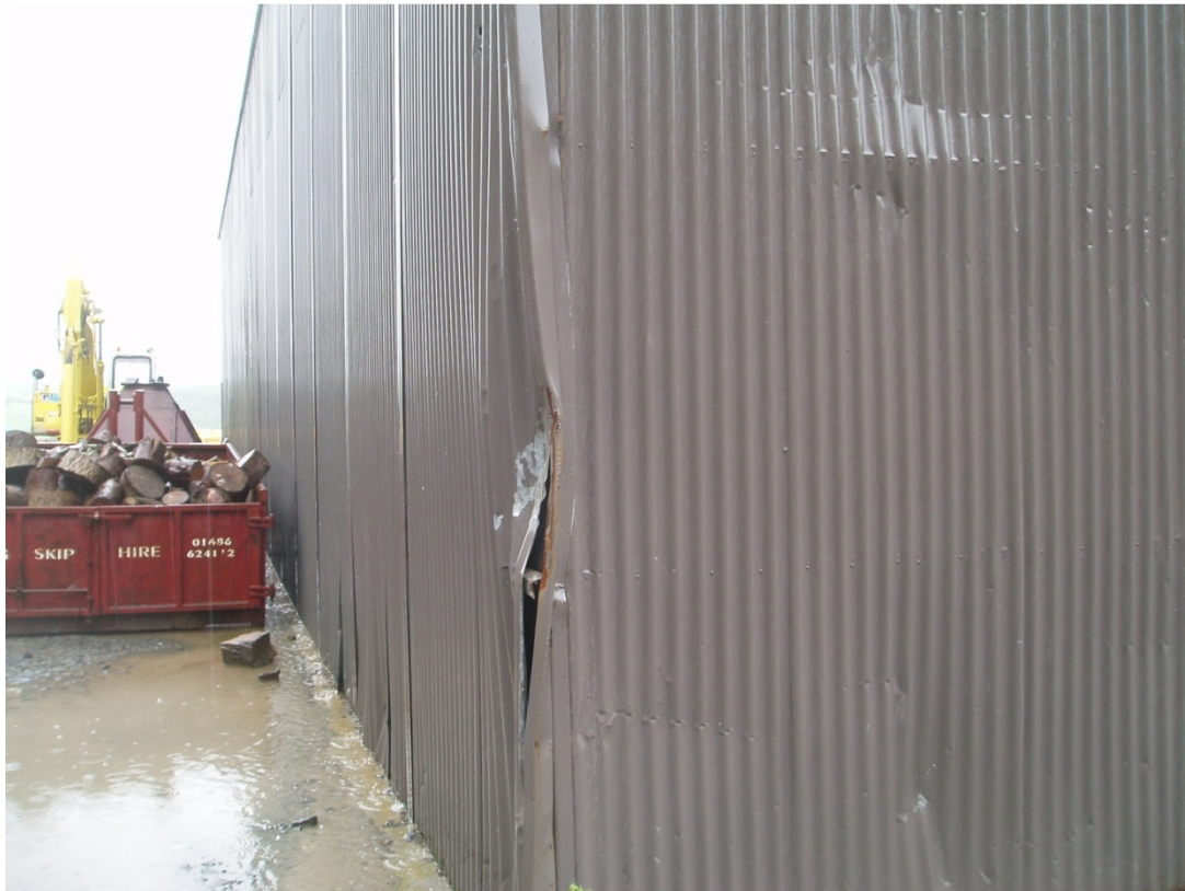
Photograph 5: Damage to existing building from rock fall
