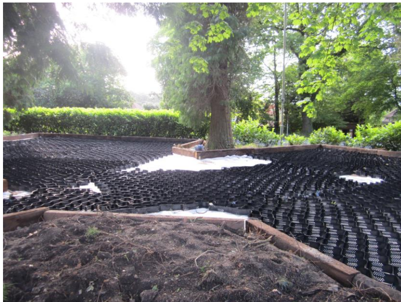
Image 6 - Cellular no-dig installation 2: A geo-textile membrane is laid across the sand bed and the cellular confinement system stretched and pinned across the surface area before being filled with no-fines aggregates.
