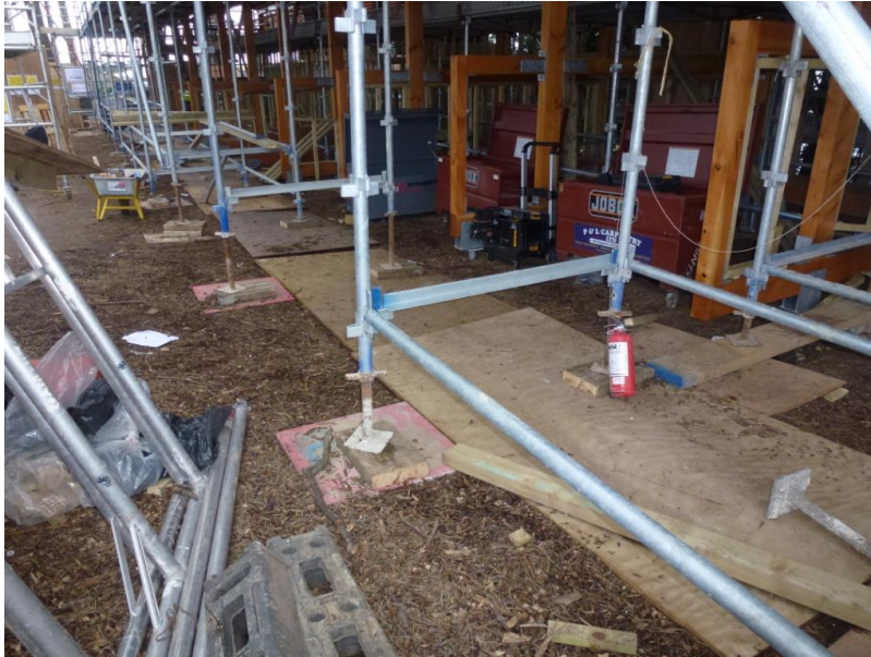
Image 9 - Scaffolding within tree protection zones: Scaffolding can be facilitated using blocks placed on ground protection to facilitate erection of the structure and pedestrian walkways without ground compaction.
