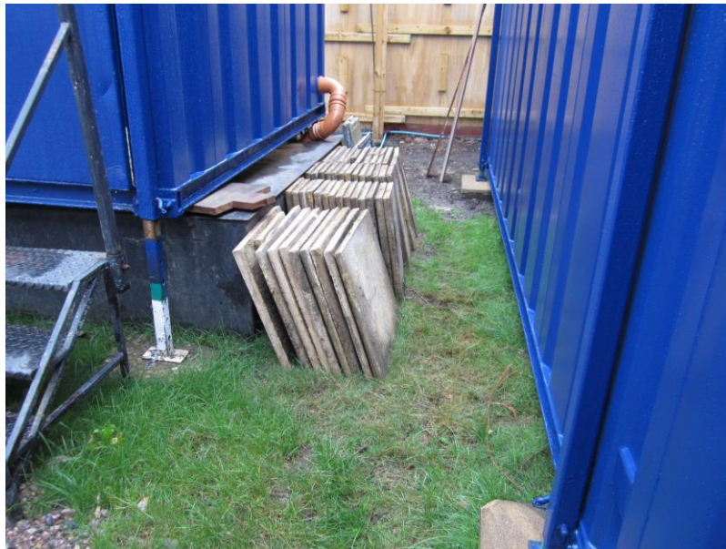
Image 5 - Containers and welfare units within RPA 1: Storage containers and welfare units may be placed and supported on above-ground structures such as pads, blocks and scaffolding.
