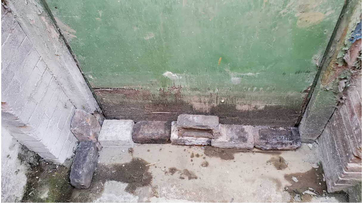
Figure 1 - bricks blocking access to basement
