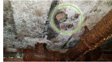
Example holes in ceiling
