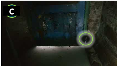
Gap at door
