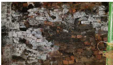
Example loose brickwork
