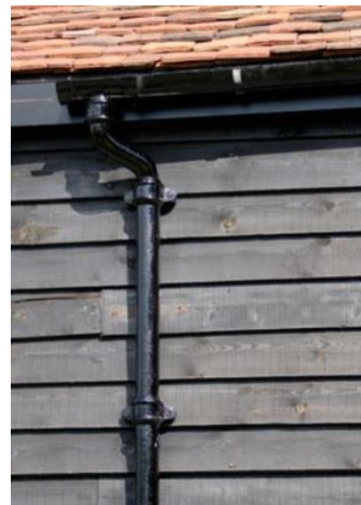
Cast iron gutters
